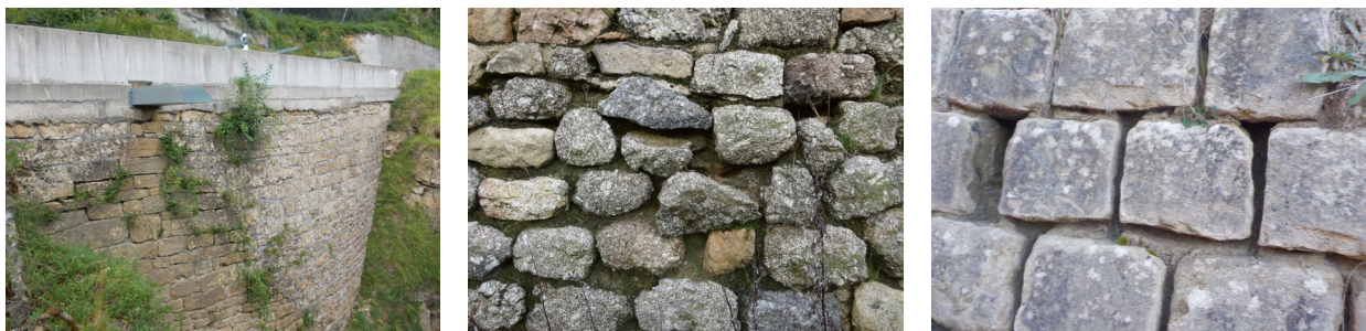
Figure 19 : Disjointoiement, altération des joints
